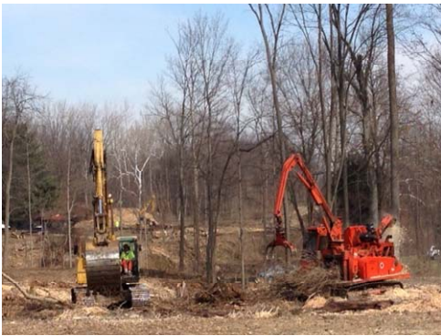
Foreman Danny Gahs and operator Blue Southard clearing right-of-way on the Illinois Street Extension project.
