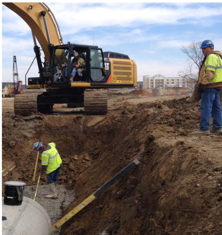
Operator Randy Certolic on one of the new Cat 336 excavators working on the US 31 project with pipe layer Tom Denning and Superintendent Roland Robinson.
