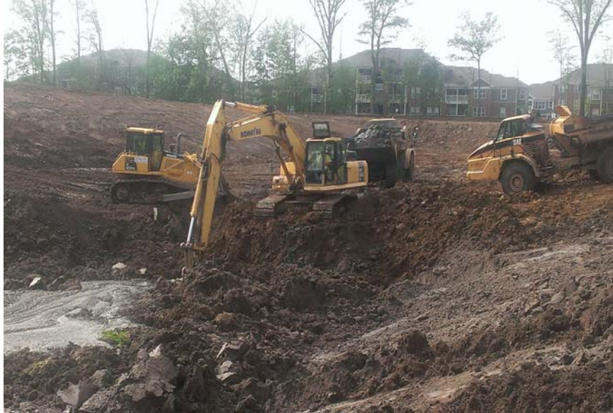
Demucking pond at Ambrose Airtech from Rob Lockhart's crew are dozer operator Mike Harden, excavator operator Royce Haste, and in the off-road trucks Nick Underhill and Kelly May. The pond has approx. 30' of fill to reach finish grade.
