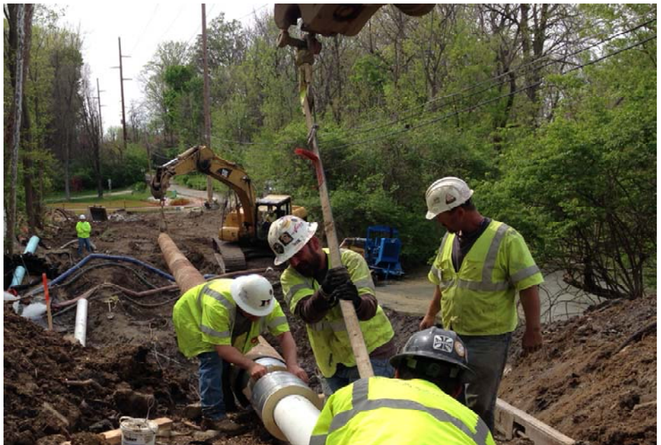
Foreman Phil Davis and crew members Troy Yeakle, Jason Haynes, Randy Davis and Duane Land (running the excavator and not pictured) are threading PVC pipe into casing preparing to cross Crooked Creek. In the background assisting on another excavator is Clint Gingerich.
