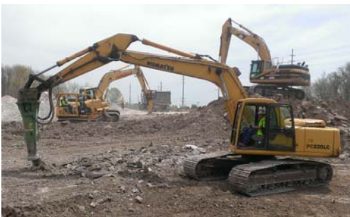
Dave Matthews, Randy Lundy, Brad Franklin, Buford Shepherd and Allen Swift on Tom Lundy's crew removing an old Prairie Concrete plant on the Worthsville Road project.
