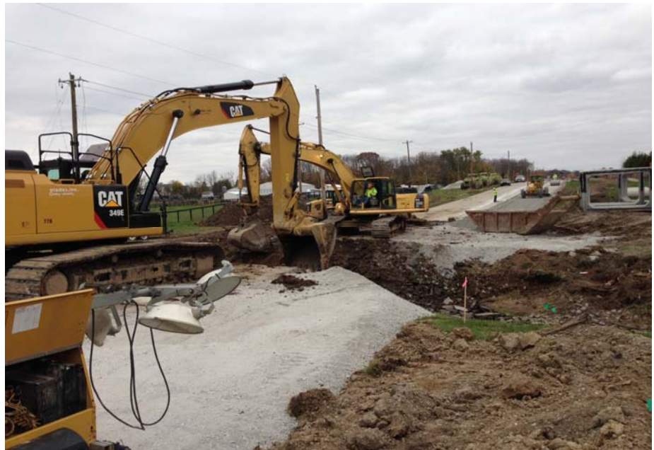
Operators Randy Certolic on CAT 349E excavator and Duane Land on Komatsu PC300 excavator excavating through 146 th Street for 8'x12' box culverts. In the background operators Chris Harris on grader and Joe Stewart on roller installing stone for temporary widening with laborer Josh Mahaney checking grade.
