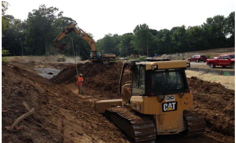
Illinois St. Extension excavating for new creek channel to redirect the flow of Williams Creek. Pictured are laborer Greg Blackburn checking grade, dozer operator Blue Southard, and working in the distance foreman Danny Gahs and operators Josh Schlabach and Richard Stewart.
