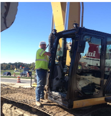
Operator Travis Koontz on US 31 cleaning the windows on one of the new 336 excavators while waiting on concrete trucks.
