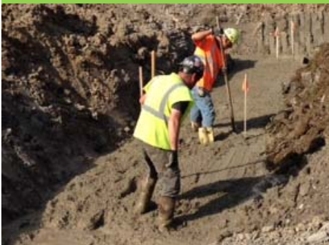
Installing mudsill for 3-sided box culvert, Illinois St., Carmel. From left to right Justin Phillips and Greg Blackburn leveling and grading lean concrete.
