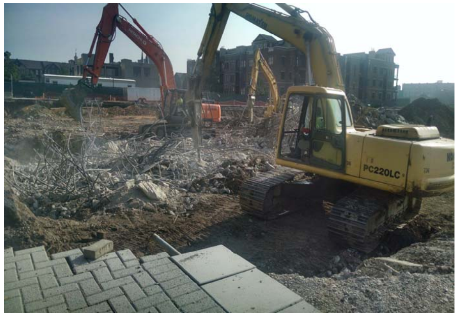
Pictured above from Tony Potter's crew are operators Dave Stewart and Juan Vasquez breaking concrete at Market Square Tower
