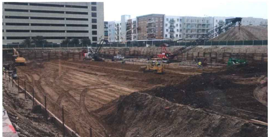
Market Square Towers project nearing completion as Tony Potter's crew works to finish site excavation.
