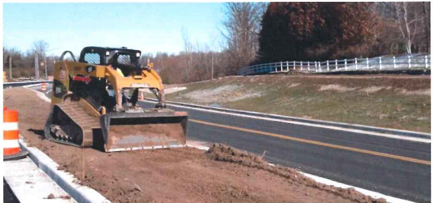
Operator Dave Kern from Shawn Smyth's crew fine grading median at Ronald Reagan Parkway in Avon.
