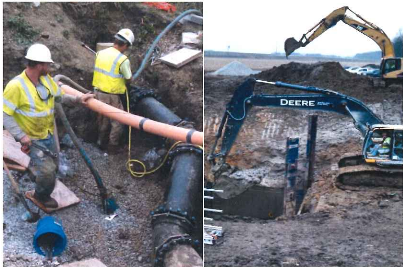
Left: Chris Odell and Scott Sours from Rob Mazur's crew installing water main under the gas main at the Indianapolis Ave. project in Lebanon. Right: Operators from Jerald Mendenhall's crew excavating for wet well on new sanitary lift station at Ronald Reagan & I-74.
